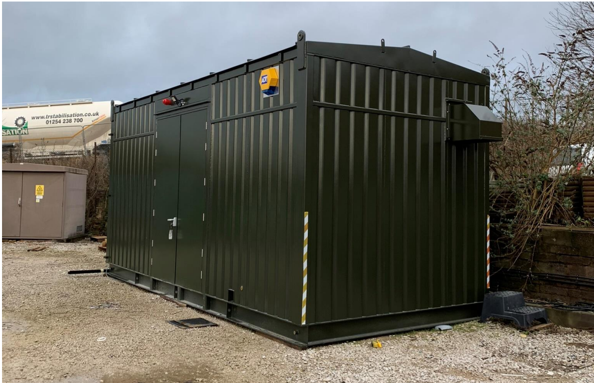
Figure 10 External view of switchgear container
