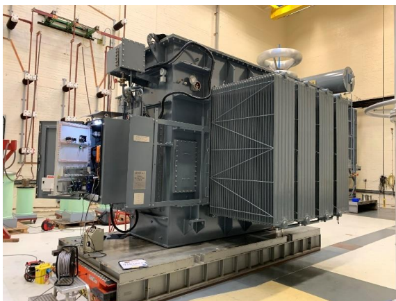
Figure 8 33/11 kV transformer in test laboratory
