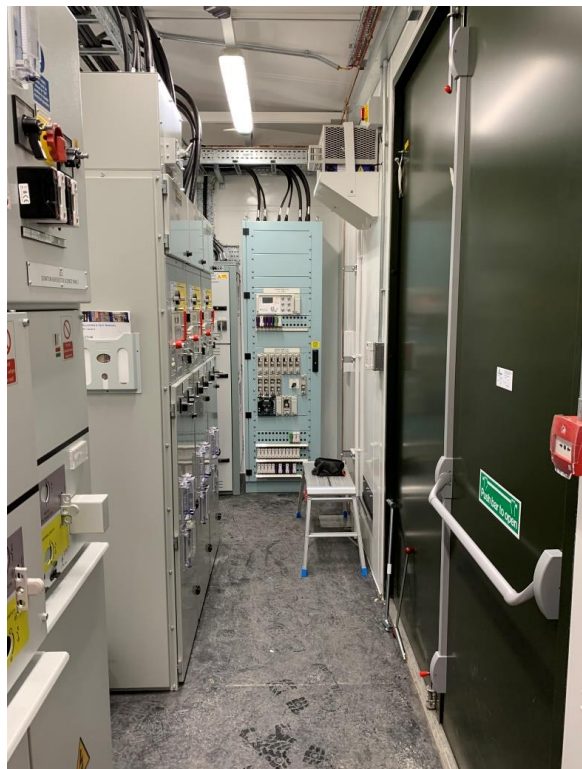
Figure 12 View of 11 kV switchgear
