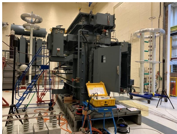
Figure 9 33/11 kV transformer undergoing tests
