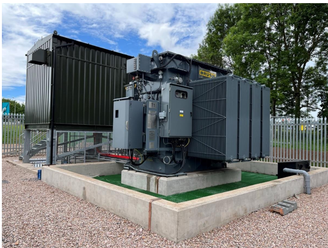
Figure 19 CCS installed and energised
