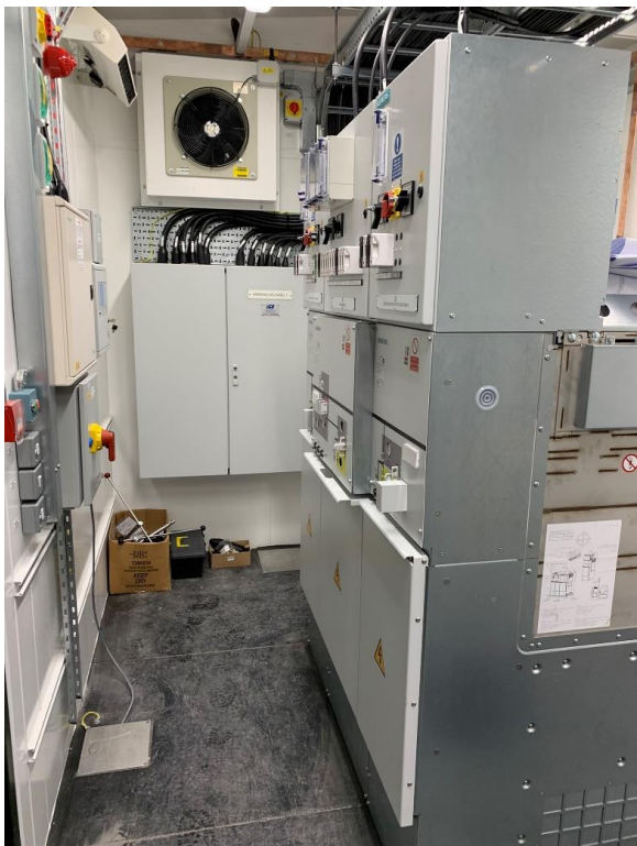
Figure 11 View of 33 kV switchgear
