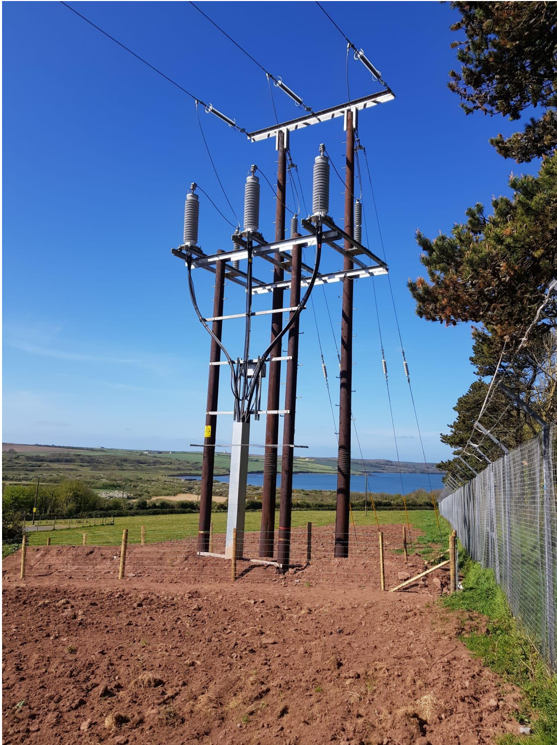
Figure 1-7 - Overhead Line to Underground Cable Terminal Connection Point (H-Pole)
