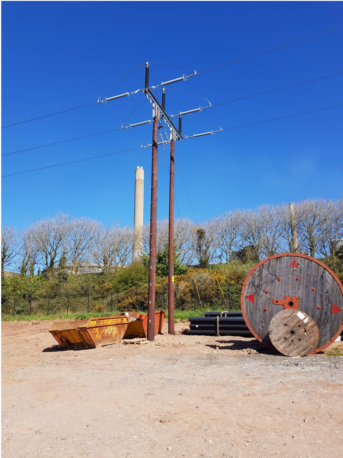
Figure 1-6 - Intermediate Overhead Line (H-Pole)
